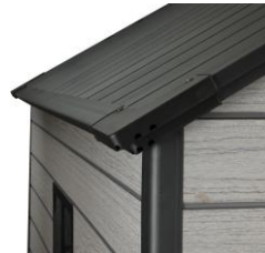
Built in Drainage
